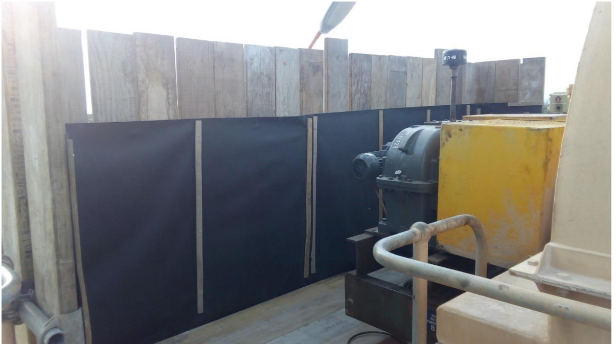
wooden barrier lined with noise attenuation fabric (Wavebar)
