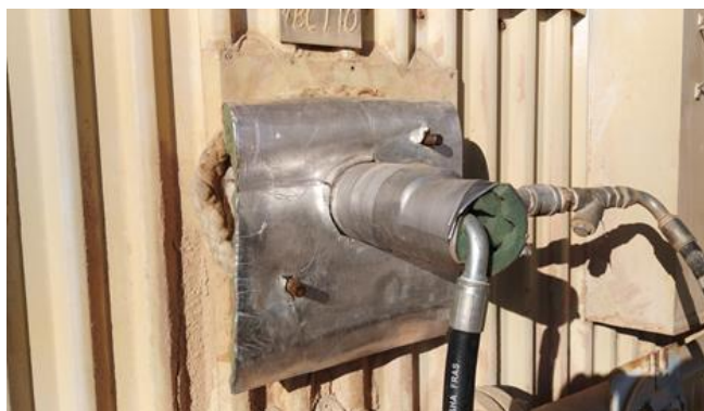
Spray nozzle lagged with Pyrotech Soundlag 4525C
