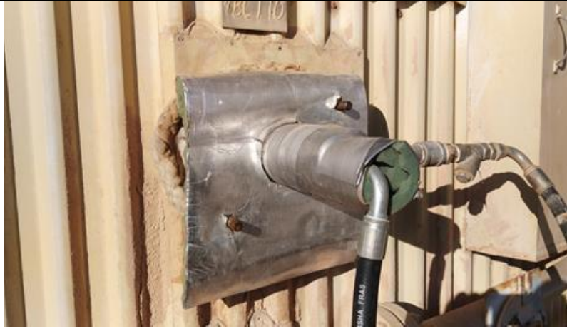
Pyrotech Soundlag 4525C installed on the spray nozzle pipework in January 2021.
