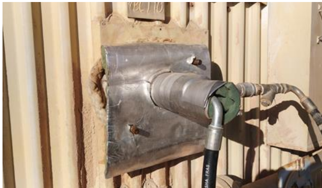
Pyrotech Soundlag 4525C installed on the spray nozzle pipework
